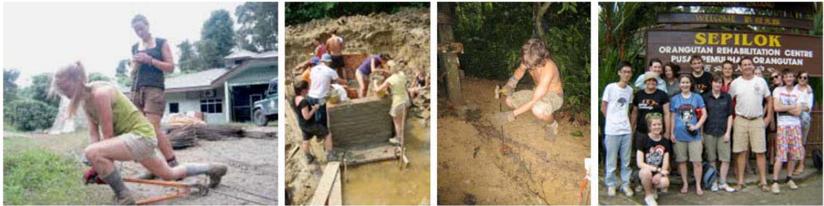
Raleigh volunteers grappling with steel rods for construction of the bear-proof fencing (left); Camps International group helping to build the Biogas Digester (centre left); BATs volunteer placing metal rods into the ground to form the base of the bear-proof fence (centre right); Wai Pak with World Challenge volunteers and BATs supervisor Howard Stanton (right).
